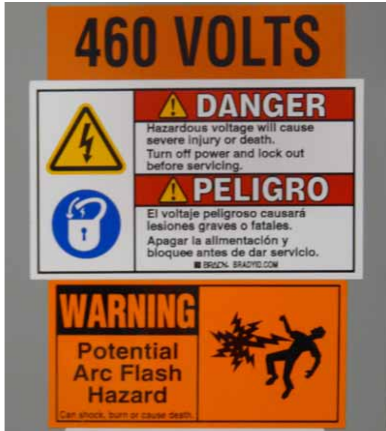
Figure 2-1. Labels on the front panel warn of electrical hazards.
