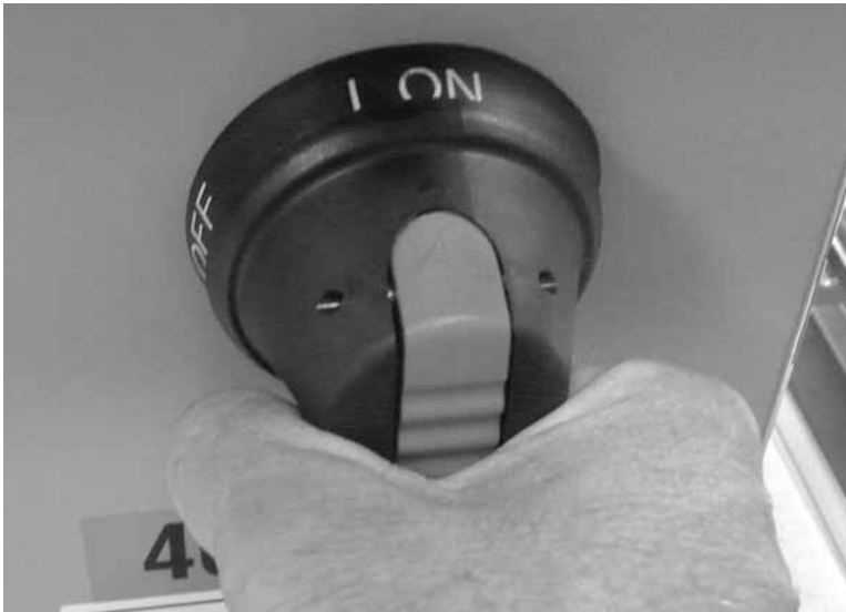
Figure 3-6. Turn the main switch on the front of the cabinet to the ON position.
