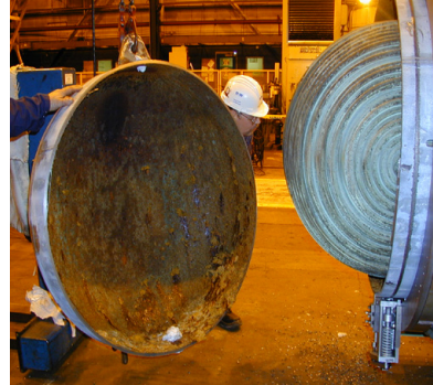
Figure 3 - Shutdown cooler with exposed tube bundle
