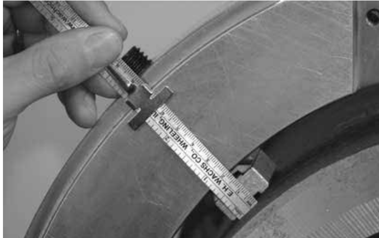
Figure 5-24. Measure the gap at the clamp leg nearest the 12 o'clock position.
