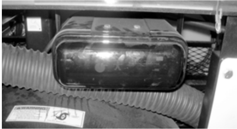
Figure 5-55. The controller for the light bar is inside a water-tight enclosure on the side of the trailer.
