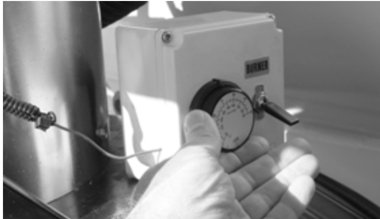
Figure 5-65. Set the water heater thermostat.
