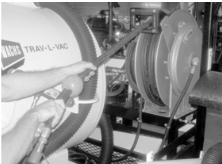
Figure 5-61. Pull the hydraulic hose pair off the hose reel to the work location.
