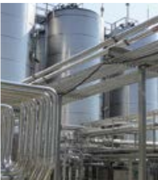
High Purity Process Pipe
