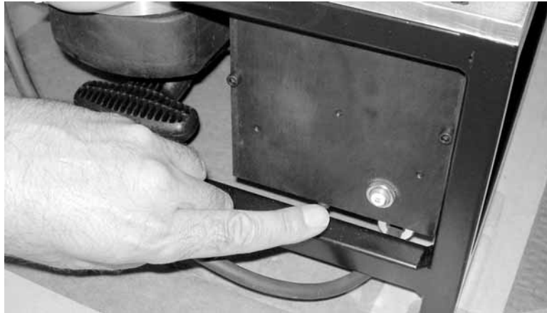
Figure 3-15. If the circuit breaker has tripped, press the button on the power supply to reset it.
