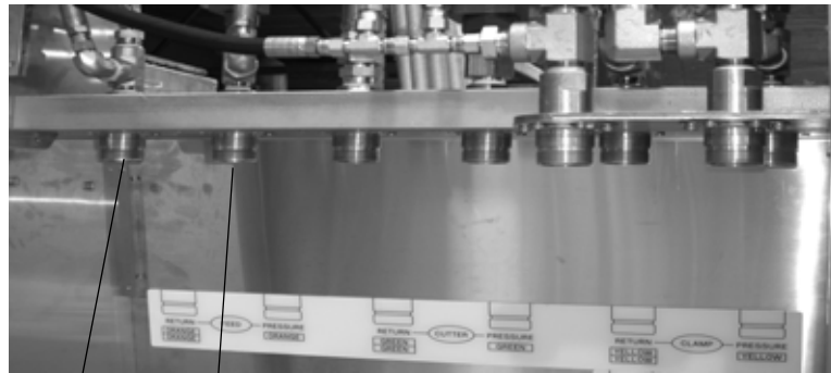
Return Pressure FEED DRIVE
