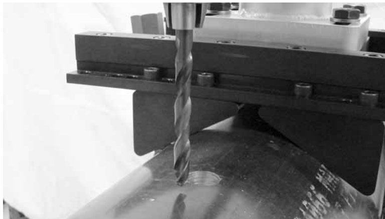
Figure 3-36. Lower the spindle and check the drill's alignment with the marked drilling location.
