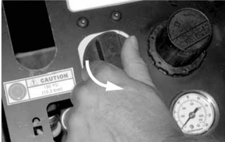
Figure 5-80. Turn the ON/OFF valve counter-clockwise to the ON position (shown in OFF position).
